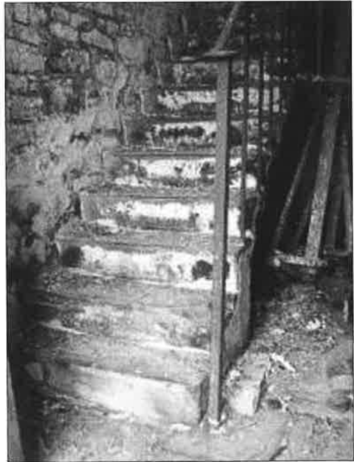
Figure 11 Borrisokane workhouse stone stairs with detailed patterned edges Source: Courtesy Brendan Treacy
