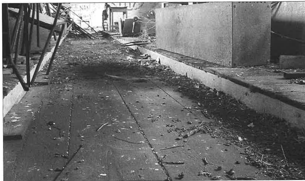
Figure 9 Borrisokane workhouse interior showing gangway in surviving dormitory flanked by sleeping platforms Source: Courtesy Brendan Treacy
